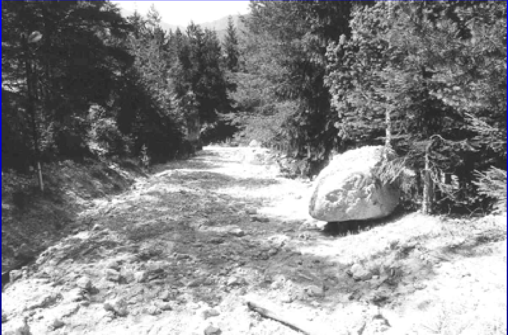
Access road to Corte full of debris. On the right a huge boulder transported by the flow (Foto: Zanfron)
